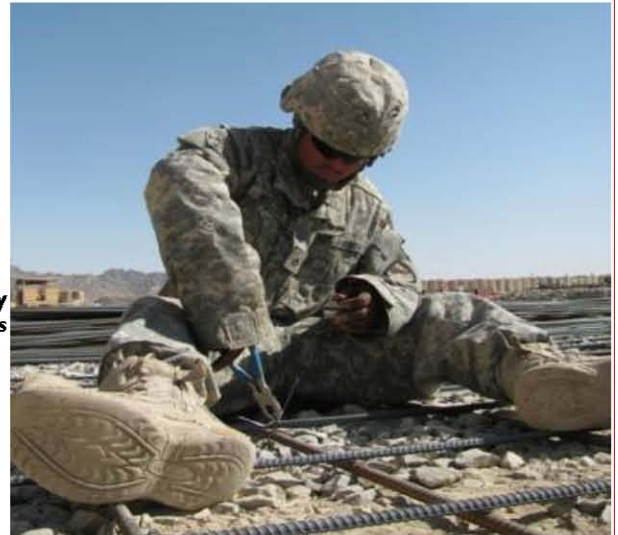
Right: PFC McClay (1st PLT) prepares the rebar for the motor pool concrete pads
