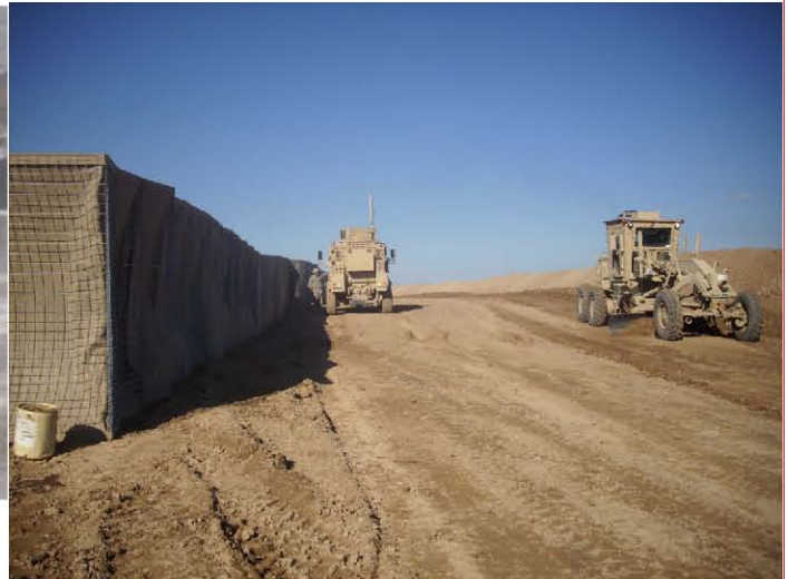
Above: 15th EN CO grading areas at FOB Delaram II in preparation for troop surge. 60th EN CO providing security for the Soldiers working.
