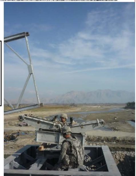
Top: 2/502nd at the Saracha Bridge Site in RC-E Middle: 2/502nd Platoon at KAF before leaving for the Saracha Bridge Mission Right: Soldiers building bridge at
