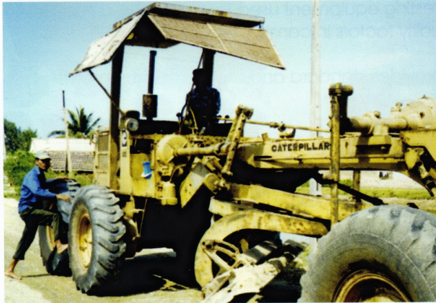
Vietnamese workers maintaining the road in 2003. Road construction was evident all along the route traveled.
