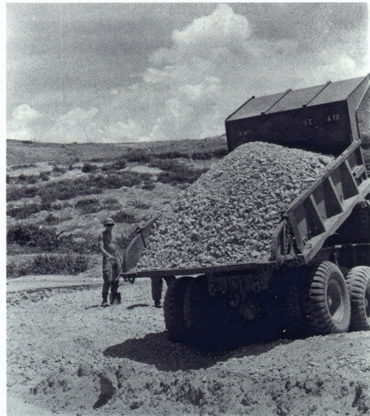
19th Engineers engaged in building QL-1 during 1969. The portion of road involved was 50 miles long with 44 bridges.
